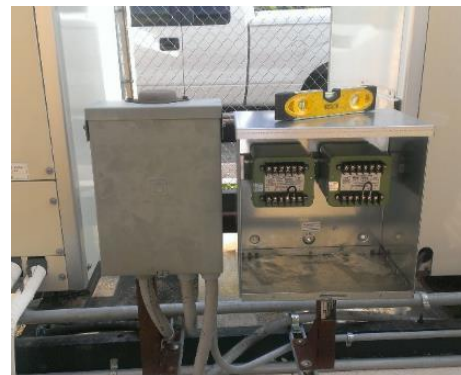
Figure 21. Wattmeters for the outdoor units
