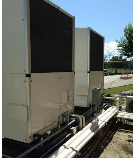
Figure 13. 8-ton units housing condenser and gas-engine
