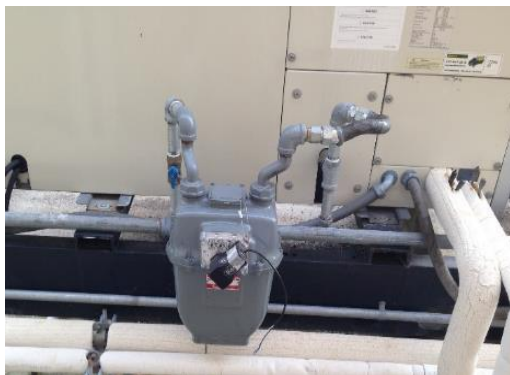
Figure 20. Natural gas consumption meter
