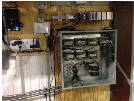
Figure 22. Wattmeters for the AHU's
