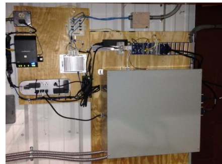
Figure 25. DAQ logging installation inside the warehouse
